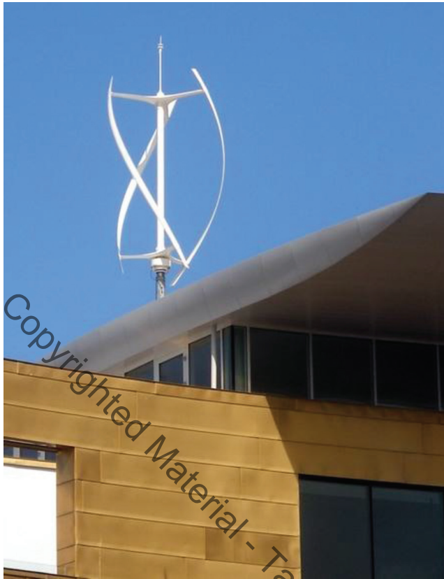
FIGURE 1.10 Small wind turbine. (Courtesy of Anders Sandberg through Wikipedia.)
