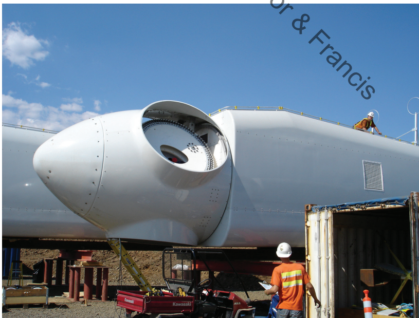
FIGURE 1.8 Nacelle of a 1.8 MW wind turbine.
